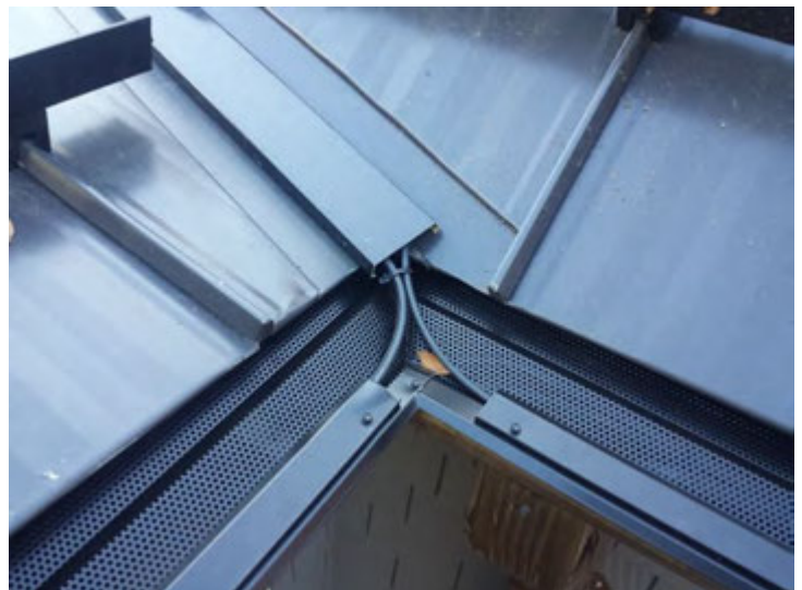
VP-MW and HGS-FE5 in Matte Black on metal standing seam roof
